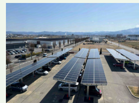
Carport-integrated solar power generation system (Tescom Denki Matsumoto Factory)
